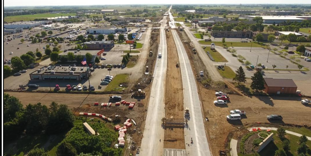
Project Photo: Work @ the intersection of 22 nd Ave (just west of 22 nd Ave...looking east)
