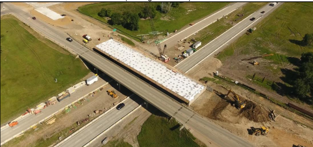
Project Photo: Bridge deck & abutment work @ the new I-29 bridge (looking northwest)
